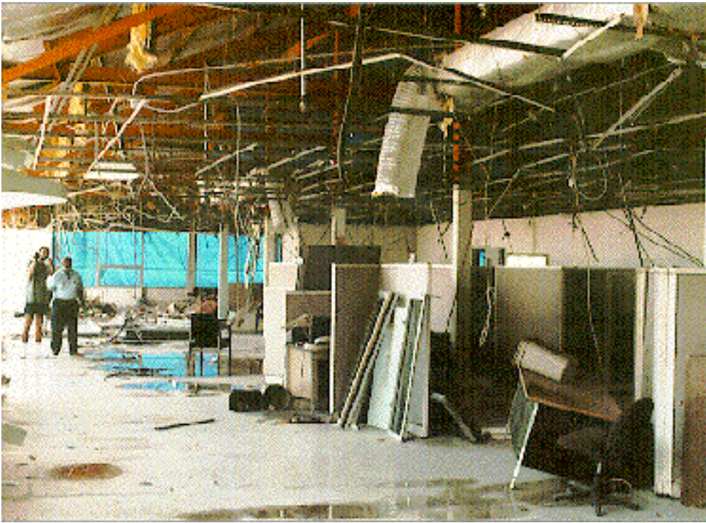
Figure 1: Condition of DPNR main offices in the wake of Hurricane Marilyn (after salvaging operations). Wall off to left of the photograph was literally blown away.
